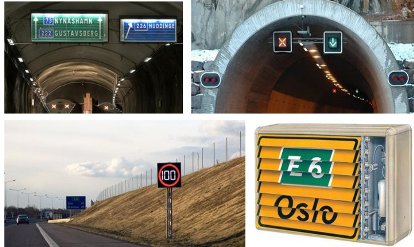
Figure 5. Safe Road's (Finland) Variable Message Sign [6]
